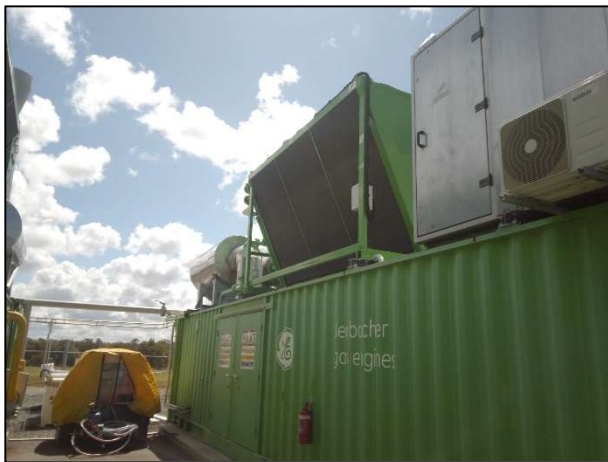
Photo 1: GE Jenbacher gas powered generator.
