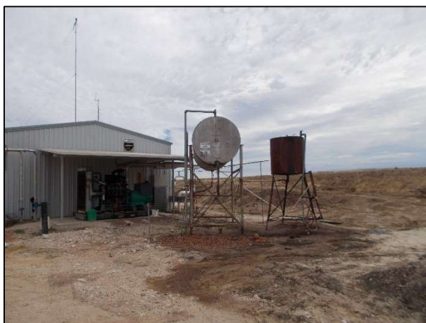
Photo 5: Bulk above ground tanks for diesel backup generators
