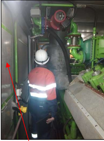
Photo 3: Thermo-acoustic panels / doors in the generator enclosure.
