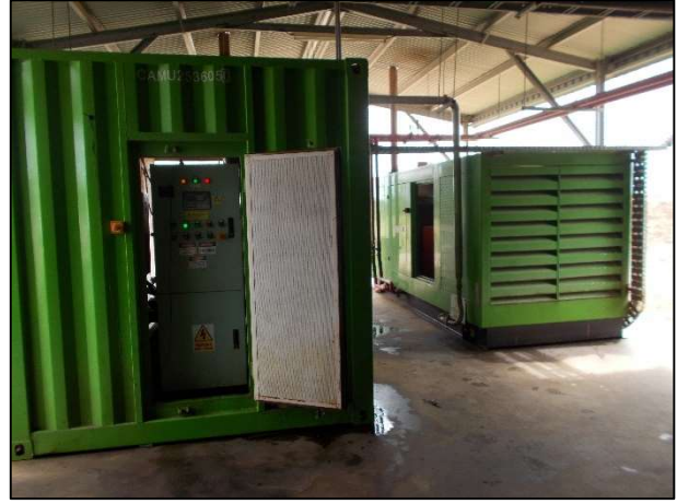
Photo 4: Generator enclosures open, to assist with cooling of the engines in hotter months.
