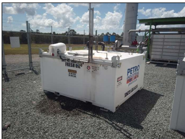
Photo 7: Bulk fresh engine oil storage with integral secondary containment.
