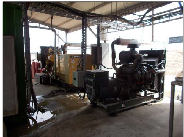
Photo 2: Open air backup generator
